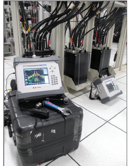
Figure 15: Telecommunications equipment room
